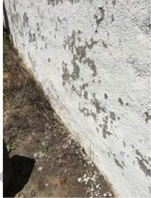
Photo 5 – Paint condition, southern face of western abutment.
